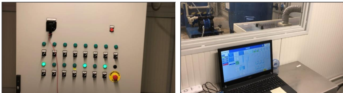
Figure 6: Pictures of the control panel area.
