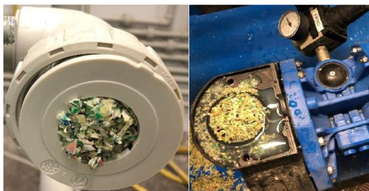
Figure 2. Photographic aspect of the pipes ( left ) and pump ( right ) clogging.
